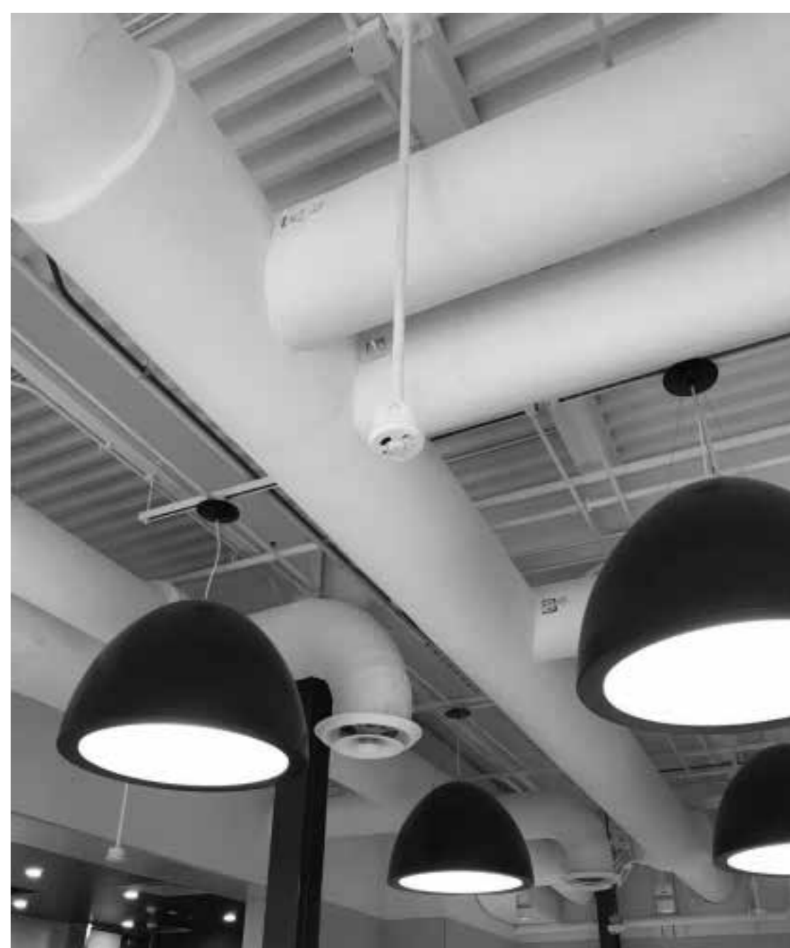
TYPICAL EXPOSED MAKE-UP-AIR ROUND DUCT
